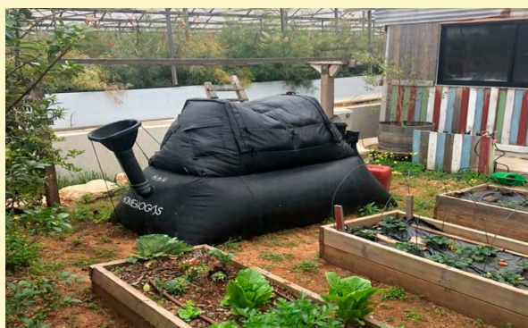
Biowaste installation in the West Bank, Palestine, producing cooking gas, electricity and fertiliser. Photo: WeEffect
