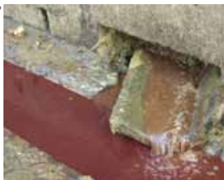
Untreated waste-water discharge from Kampala abattoir.
