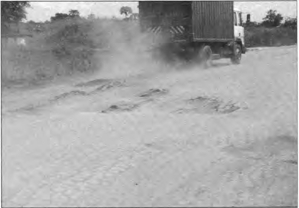
Due to lack of maintenance, the roads in Tanzania are in poor shape. Rehabilitation today will cost more than three times what regular maintenance would have cost. Photo: Tage Klingberg.
