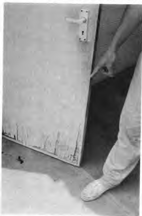
In need of maintenance.
