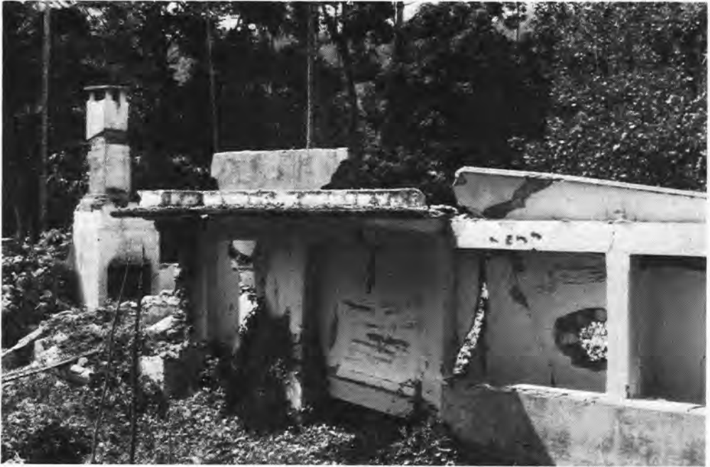
16. Collapsed house at Pahalagammedda, Niyangandora. The damage is stated to have occurred in 1986. This area is badly affected by slides and soil creep, and all houses werw abandoned by January 19, 1988.
