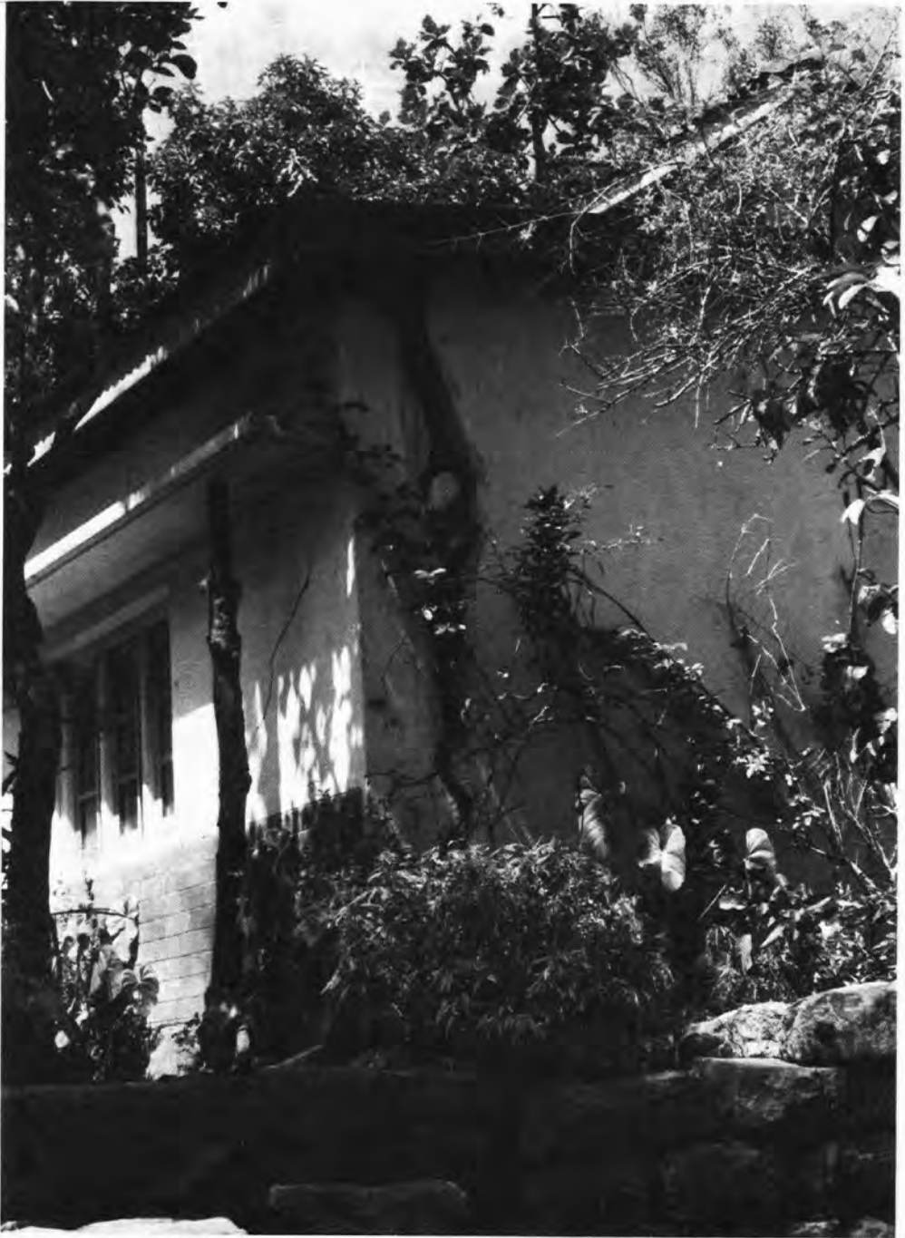
14. Deep cracks across the wall and floor of a house at Wataddora, January 17, 1988. The cracks run parallel to the slope and the reservoir shore line.
