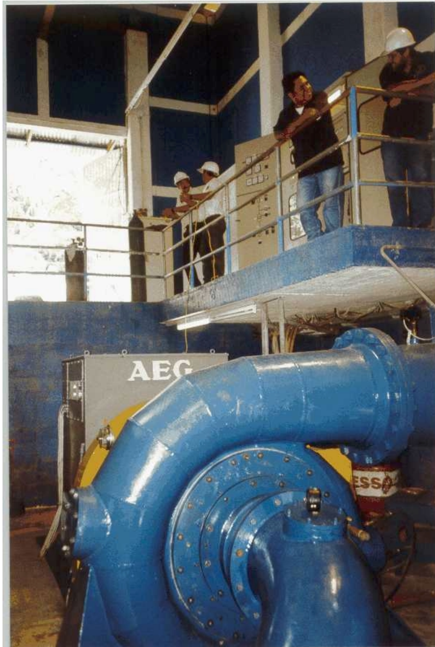
Photo: Wabule turbine and generator
