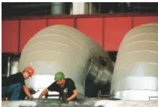
Lithuanian district heating plant.
