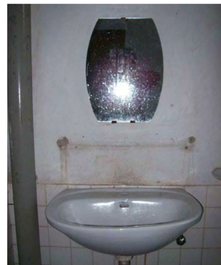
This sink is in a new District hospital. It is the only washing facility for out-patients and yet it has not been plumbed in.
