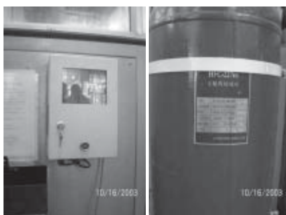
Fig. 4.5 Flame Monitor & extinguisher at Cosmopolitan
