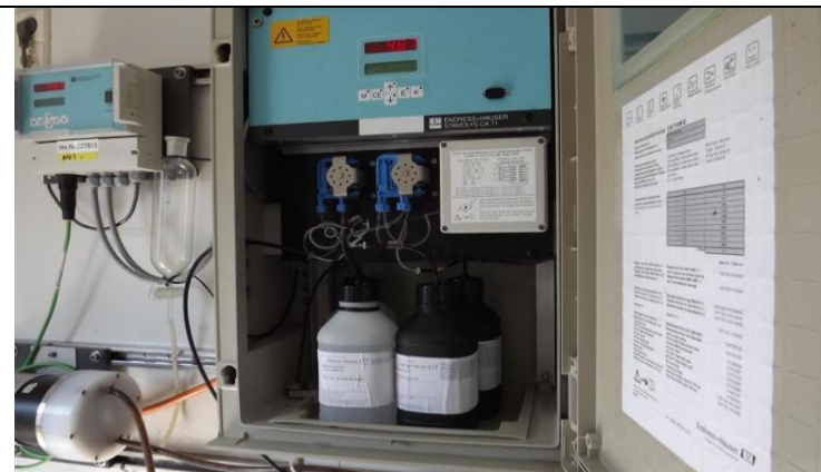
The picture above shows the online measurement used for the plant process control to secure high efficiency of the treatment. Installed at the 2 nd phase
