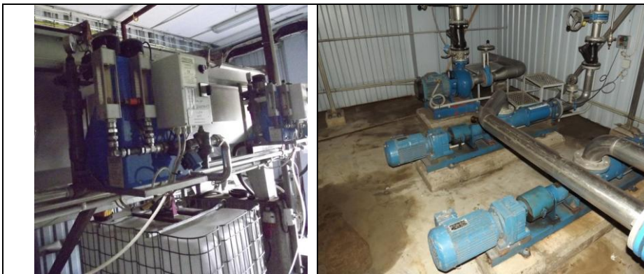
The pictures above show the polymer unit and sludge pumps in dewatering building. Most of mechanical equipment supplied from Sweden. Condition of the equipment is still good.
