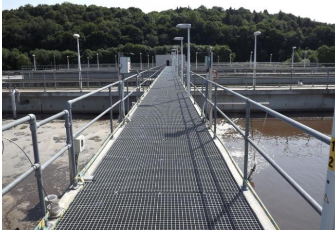
The picture above shows the activated sludge tank constructed in the 2 nd phase.
