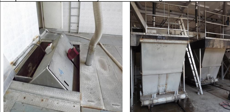
The pictures above show the mechanical treatment equipment supplied through Sida support: screens and sand containers, which have been operating from 1999.
