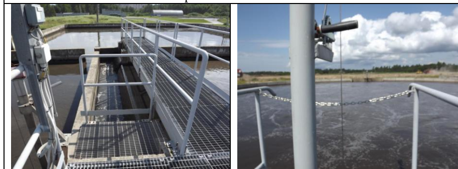
The pictures above show P removal tank and activated sludge tank. Condition of process units is good.
