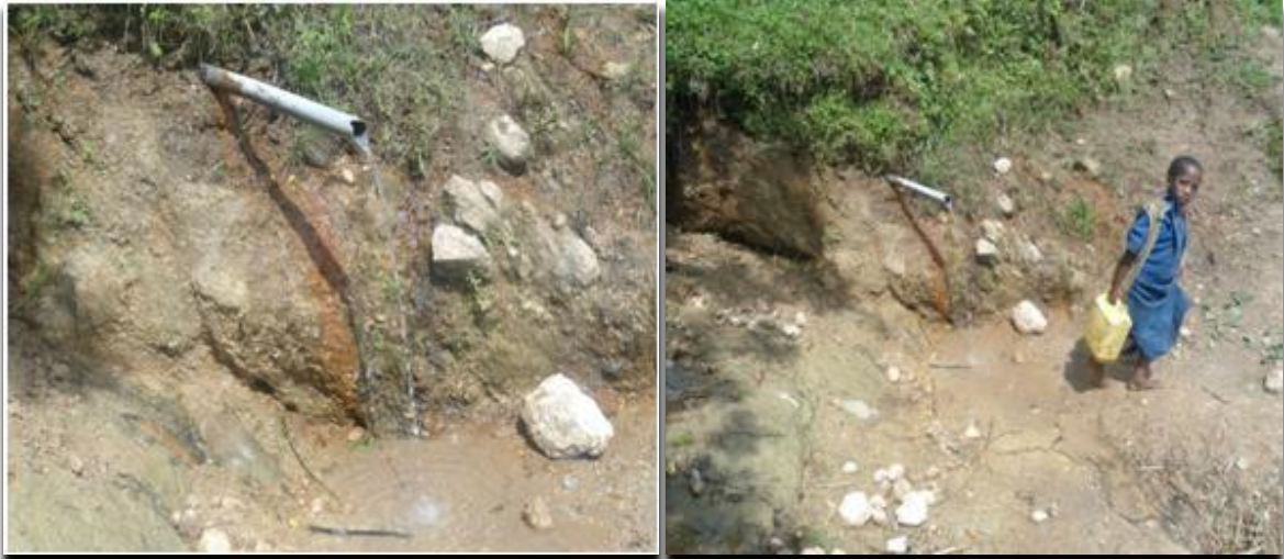
The PVC pipe capturing water that used to flow in different directions
