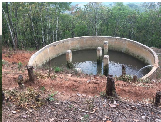
Reservoir that needs a roof
